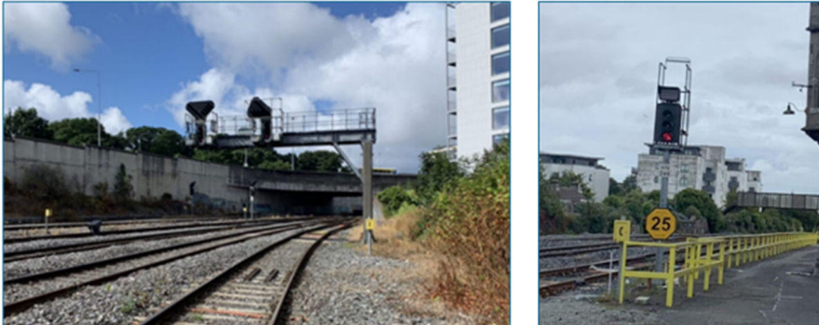
Figure 4-19 Typical Existing Signalling Infrastructure
